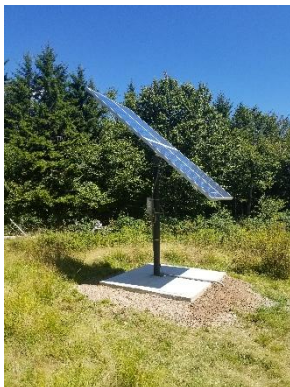
Remote Site Solar Installation
