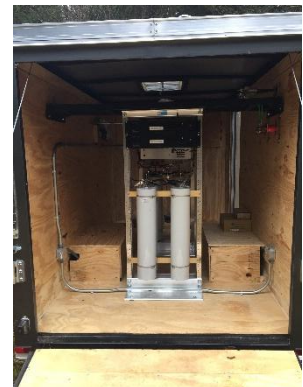
Mobile Radio Repeater Build-out
